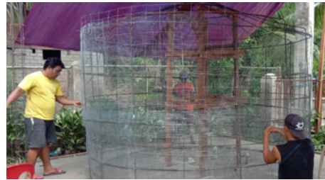
A rainwater storage tank (November 2019)
