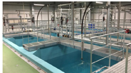
FRD Japan commercial plant (in Kisarazu City)
