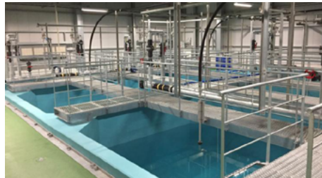
FRD Japan commercial plant (in Kisarazu City)
