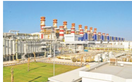
The Ras Laffan C water desalination plant
