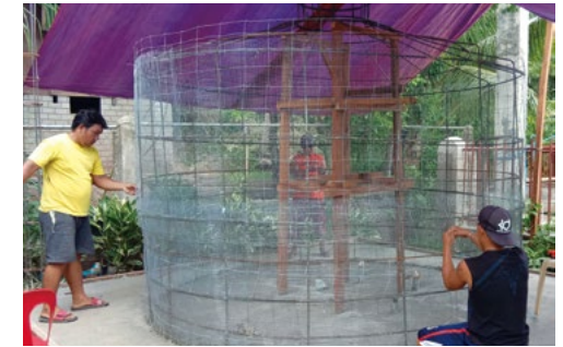
A rainwater storage tank (November 2019)
