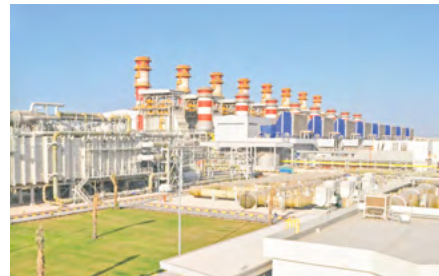
The Ras Laffan C water desalination plant
