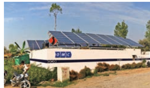
Small solar power generator installed in non-electrified areas in India
