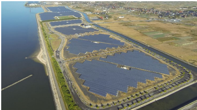
Solar Power Generation Business (Tottori Yonago Solar Park)
