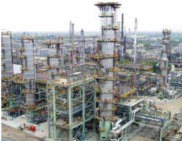
A currently operating LAB plant with a similar design
