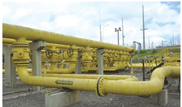
Gas distribution station
