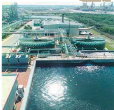
Water treatment facility, Atlatec
